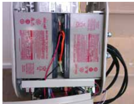
BATTERIES ROTATE BACK IN PLACE
